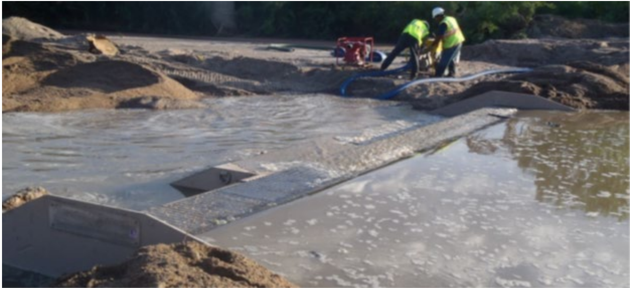
Figure 4.22 Sediment Collector™ Installed in Fountain Creek, CO (Tucker et al., 2015)
