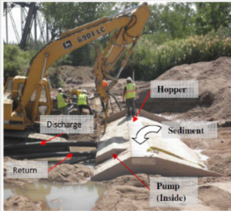
Components of the Sediment Collector™ at the Fountain Creek, Colo., installation. (Tucker et al., 2015)
